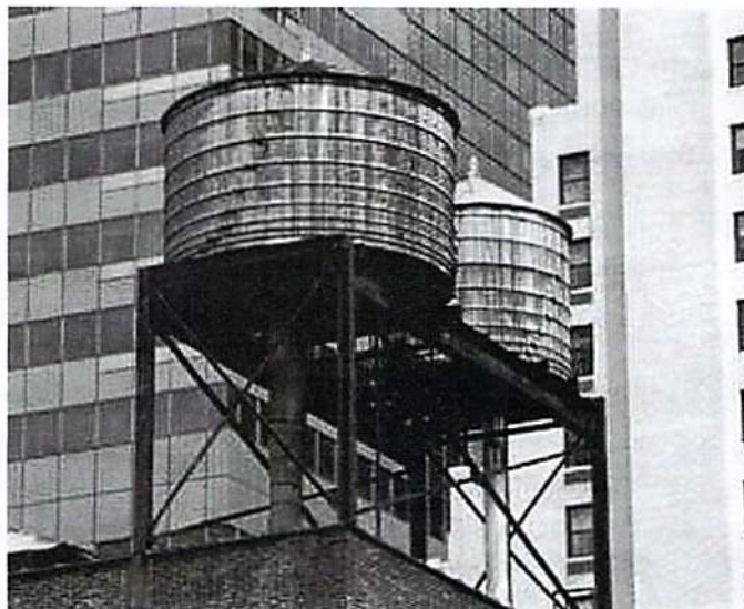
High Rise Building Roof Water Reservoir
